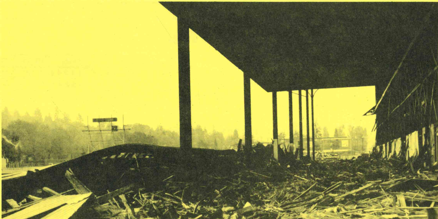
West Grandstand of Hayward Field was condemned and razed this fall. More than $600,000 has been donated for a new facility. Bill Bowerman and the Hayward Field Restoration Committee need about $300,000 more for mini-field house and grandstand. New facility will insure more major meets in State of Oregon.
